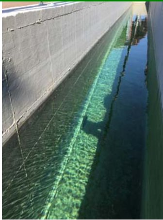
Camera effluente – Acqua chiarificata Effluent chamber – Clarified water
